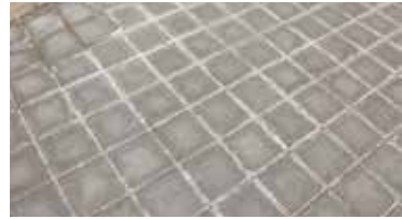
Over salted pavers
